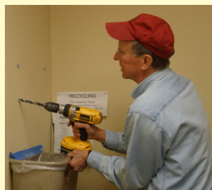
Right: Volunteer Tony Zornik drills holes to mount a shelf in the new Idaho AEYC kitchen area.
